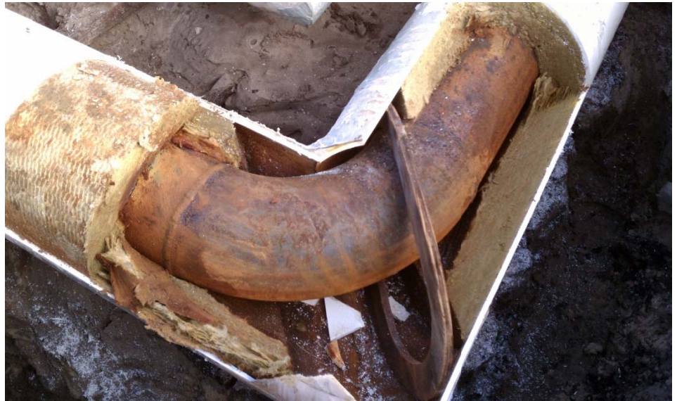
Figure 1 The existing site piping was inspected and found to be in good condition.
